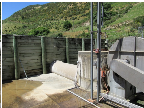
BIOFILTER INFEED DUCT FROM FAN
